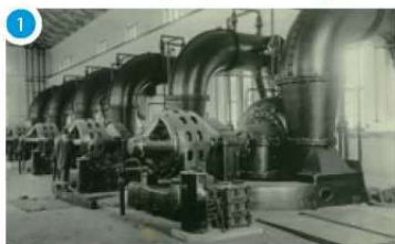
Tokyo's Asakusa Tamachi pump station
